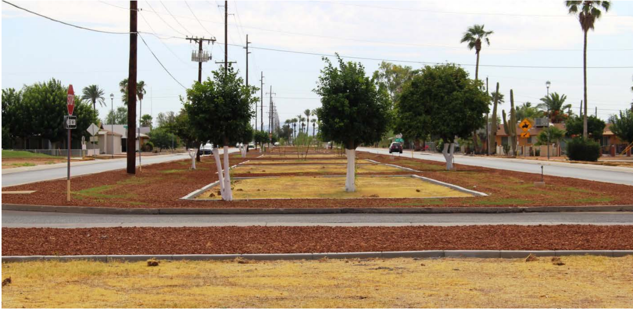
MCDOT Roadway Median Landscape Conversion Project Underway on Alabama Avenue east of 111 th Avenue
